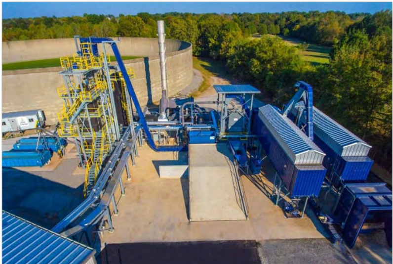
Photograph 2-4 Woody Biomass Downdraft Gasifier Facility in Lebanon, Tennessee
